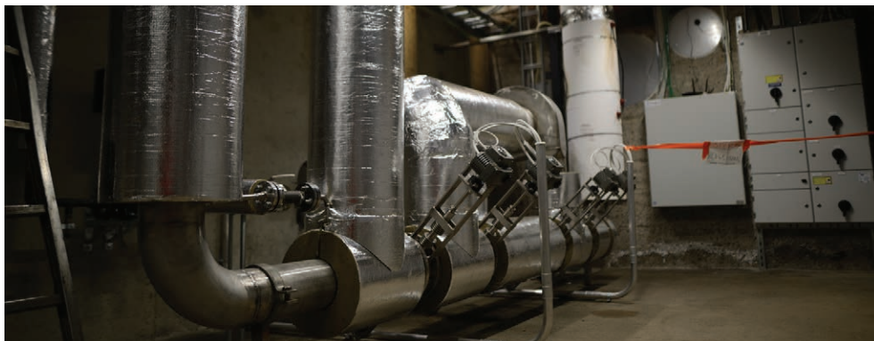
FIGURE 7 Part of the heat transfer system installed by Polar Night Energy in Tampere, Finland. The vertical pipes at left are part of the heat exchanger, while the resistive heater elements are wrapped in white insulation at right. Between these components is the air-circulating radial blower.
