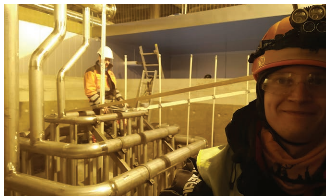
FIGURE 4 Tommi Eronen (foreground) and Ylönen inspecting the ductwork of a Polar Night Energy heat storage vessel.
